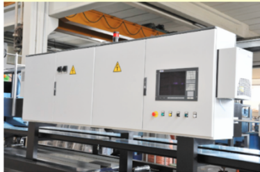
Main Electric control board
